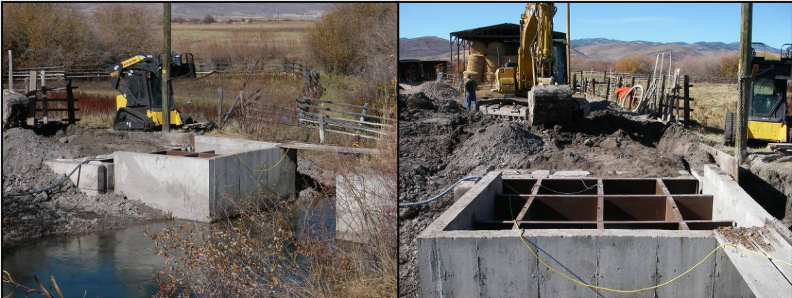
Transtrum Irrigation Diversion during construction. The new fish ladder (right) sits inside the existing diversion abutment (left). This configuration allows for upstream fish passage without significantly increasing the footprint of the existing structure.
