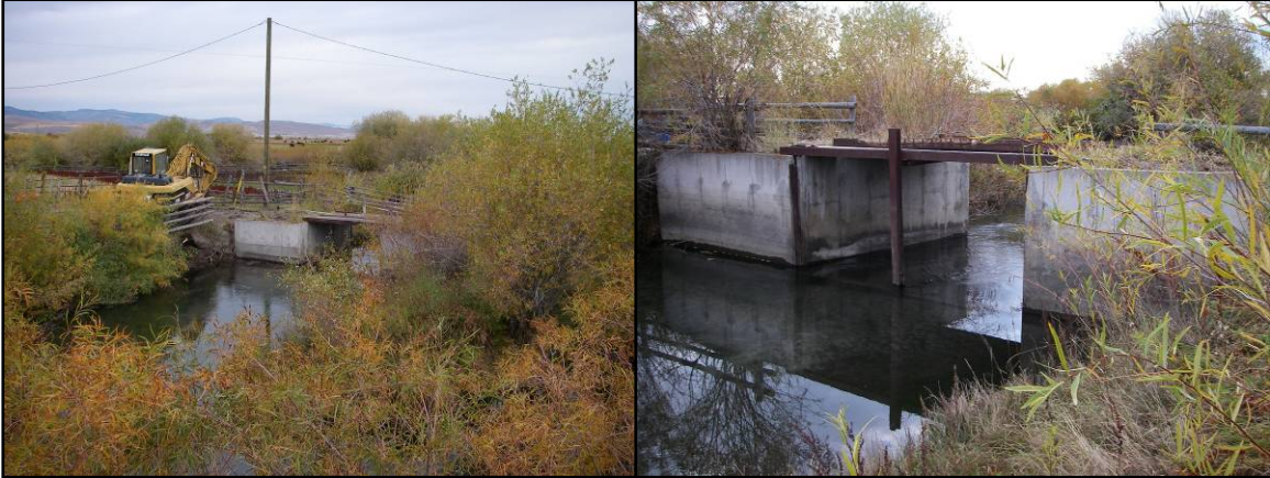
Transtrum Irrigation Diversion before fish passage restoration, as viewed from downstream (left) and upstream (right).
