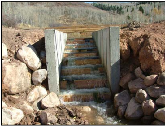
Figure 2: New fish ladders constructed on both ponds with wooden steps in place.
