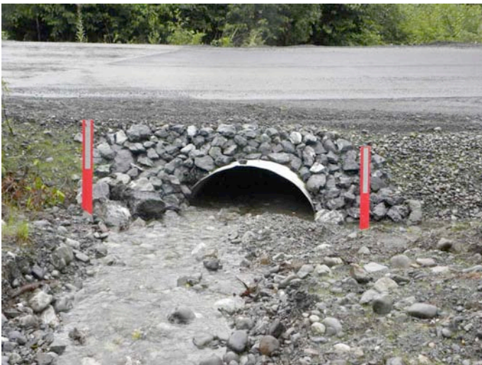
Figure 10: Looking west (downstream) at the upstream side of the Whiskey Creek culvert.
