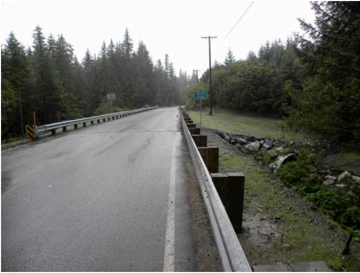
Figure 3: Looking north at Eccles Creek crossing from the north end of SE retaining wall.
