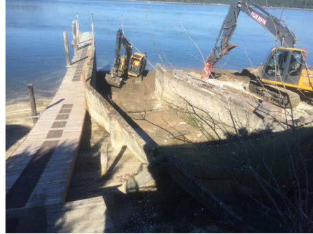
Demolition is underway at the Collier boat ramp and jetty site. Photo credit: Rich Carlson, USFWS
