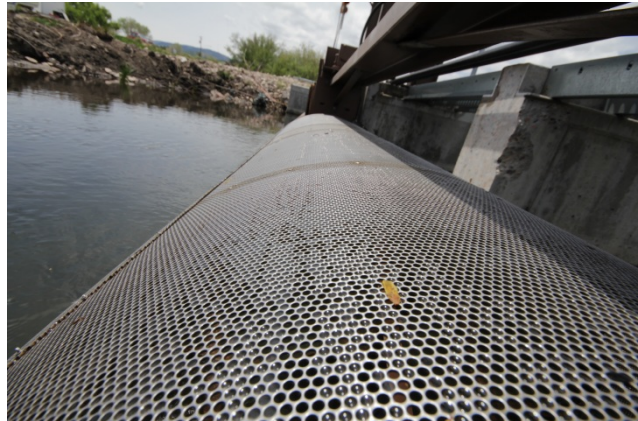
Photo 3: A close-up of the new rotary drum screens.
