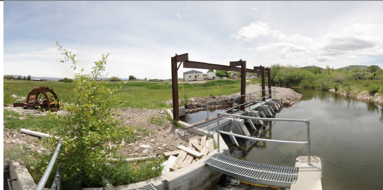
Photo 5: Island Diversion in operation on 6/6/2012. A few minor project components were completed after this photo was taken. A video of this diversion project can be viewed at: http://youtu.be/KvvS0fnzsgg .
