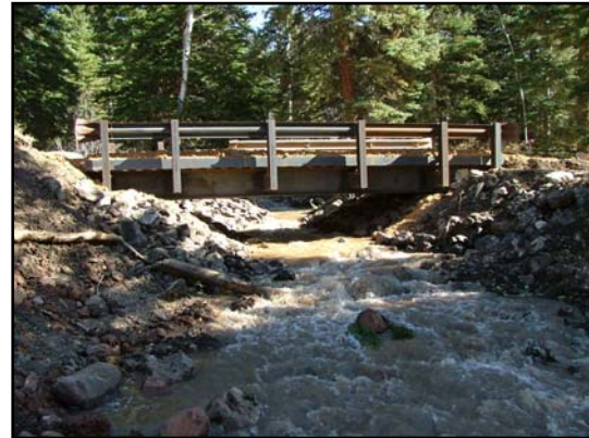
Figure 3: A new bridge, which has replaced a previously existing culvert that was considered a partial fish migration barrier.
