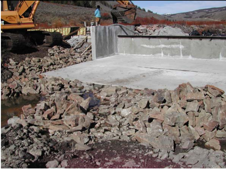
During construction, showing the concrete splash pad and wing walls installed in the low flow notch. Photo taken October 2006.
