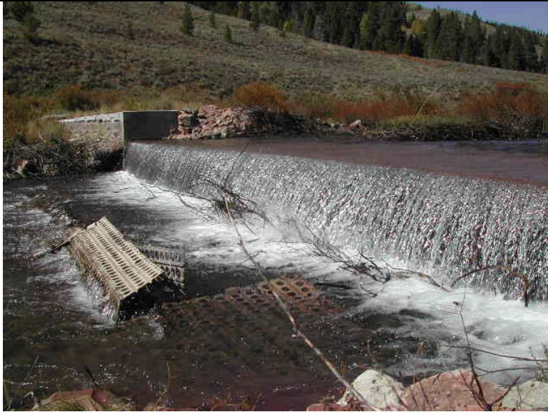
Barrier before construction. Splash pad created from metal landing mats in place to prevent development of jump pool have been torn up by flow and icing. Photo taken October 2005.
