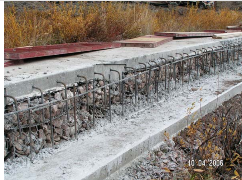
Concrete cap on gabions, work ongoing to put concrete cap on downstream face of barrier. Photo taken October 2006.
