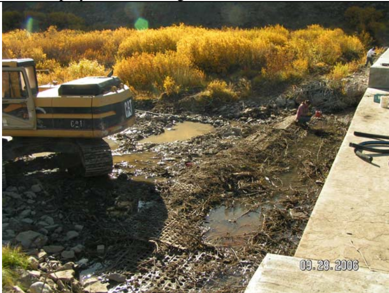
Start of construction, metal landing mat splash pad being removed. Photo taken September 2006.
